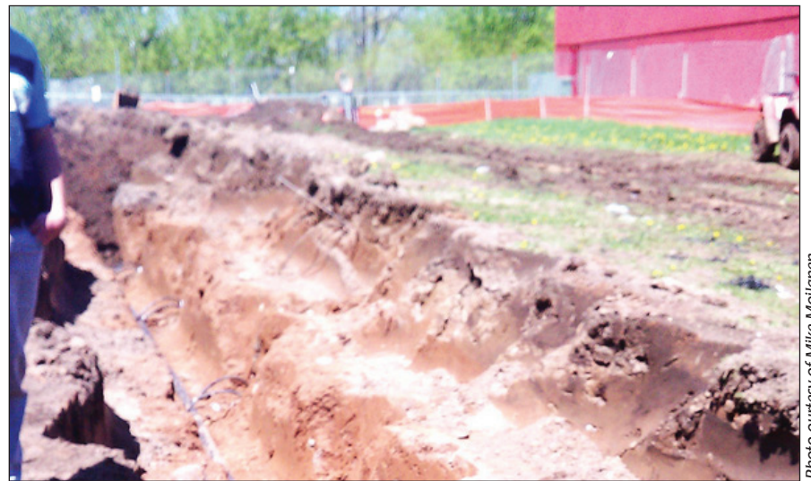
The underground pipe pictured above is a part of the early education building's geothermal heating and cooling system.
